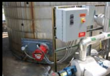
Separation tank heater.
