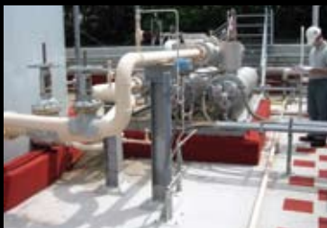
Gas transmission heater.
