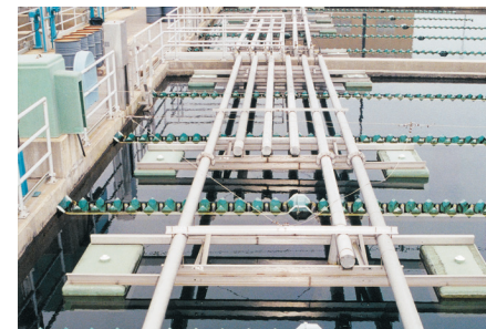
Water & Wastewater Treatment
